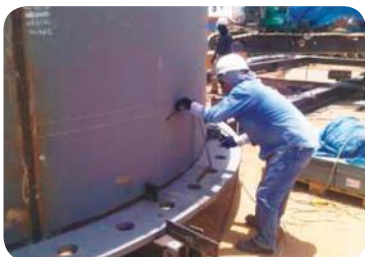
10 Feature Project: Main and Bypass stack at Dhurma, Riyadh
